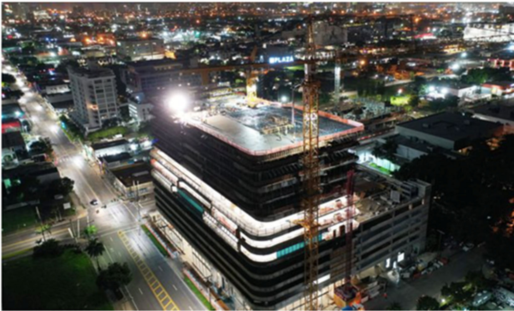
An aerial photo of The Gateway at Wynwood office building under construction in Miami's Wynwood Arts District. Courtesy photo
